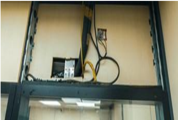
Concealed AC Ducting And Drainage
